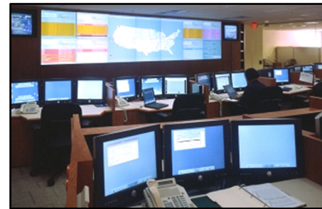
Network Operations Center (NOC)
