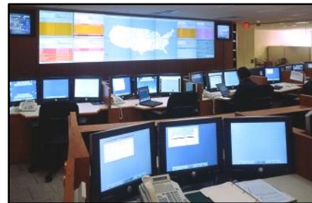
Network Operations Center (NOC)
